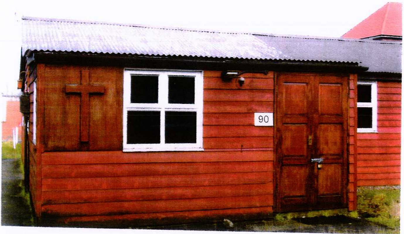
Former Garrison Church dedicated to St. Michael and St. Nicholas. This wooden building was there in 1948 as a 'chapel', but former Chief Petty Officer Kathleen O'Kane states that it was there during the Second World War. It is numbered 90 on the EHS plan. (A.J. Malley)
